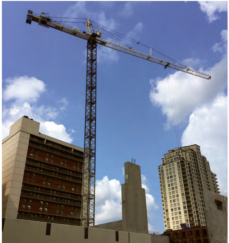
Joe Soares Jr. is operating a Terex Peiner SK415 Tower Crane, building a 24-storey residential high rise for Tricar Developments in downtown London.
