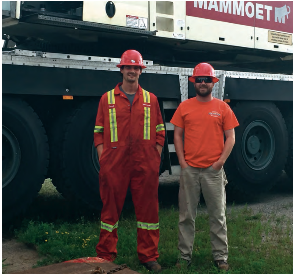
L to R: Local 793 crane operator Andrew Burgess and apprentice Jacob Murphy working at the West Nipissing electric dam removing the original turbines built in 1920 with an AC 350t Terex Demag.
