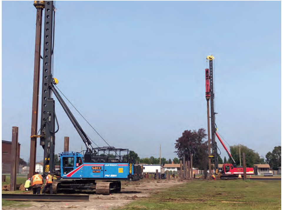
Sacchetti Construction operators doing piling operations at the new Thunder Bay public school worth $20 million. Matt Whitney and Kelan Hartviksen are at the controls of the Junttan pile driving rigs. They are driving 280 piles, to an average depth of 160 feet.
