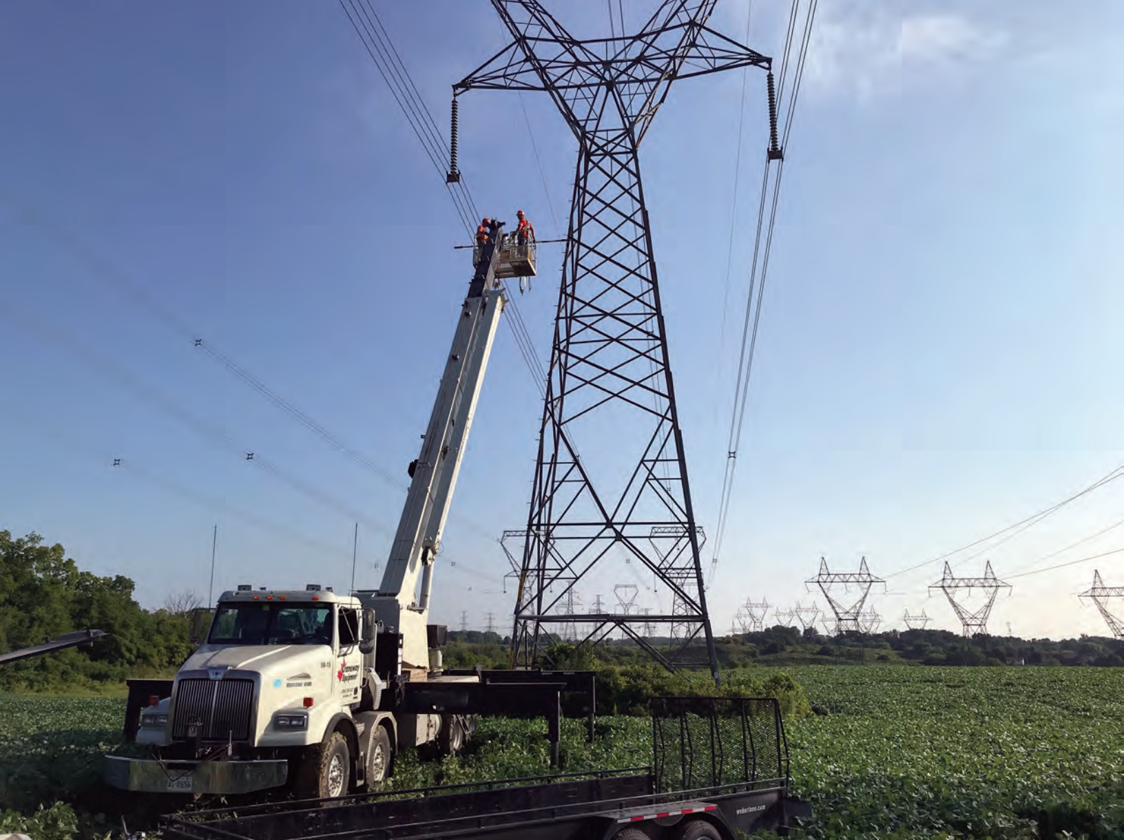
Operator Mike Higgins working for Craneway on a 45-ton national crane west of Caledonia on the N580M line. The work being done is part of a series of line work changing insulators.
